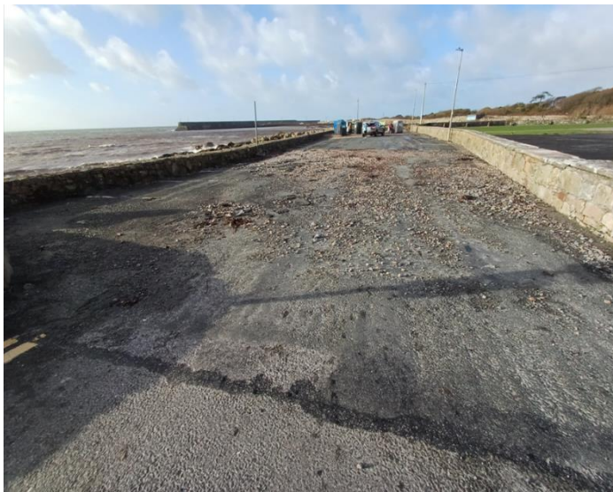
AN SPIDÉAL PROMENADE- STORM ASHLEY DAMAGE
