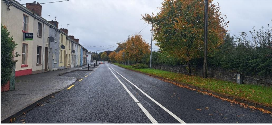
RI PROJECT WORK AT POLLBOY BEING COMPLETED, INCLUDING REINSTATEMENT OF IRONWORKS AND ROAD MARKINGS
