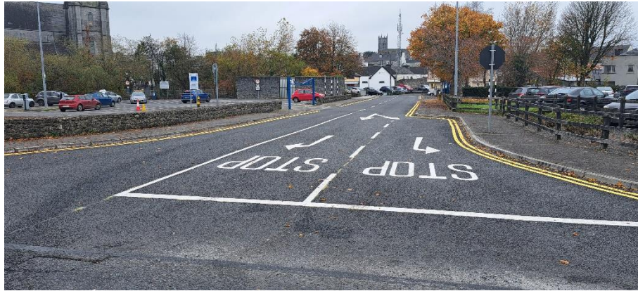
RI PROJECT WORK COMPLETED AT TOWNPARKS, BALLINASLOE, INCLUDING DRAINAGE IMPROVEMENTS IN ADVANCE
