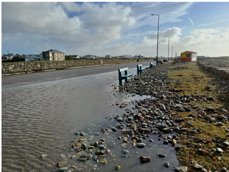
AN SPIDÉAL PROMENADE- STORM ASHLEY DAMAGE
