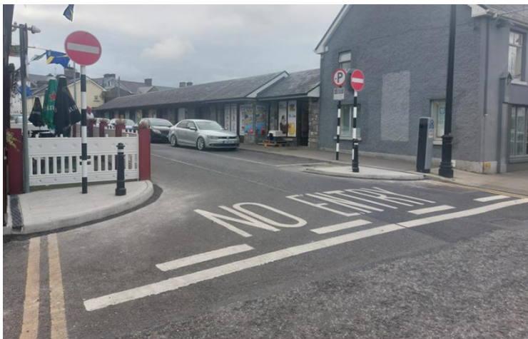
INTRODUCTION OF NEW BUILD OUTS AT KING STREET, LOUGHREA UNDER THE LOW-COST SAFETY IMPROVEMENT SCHEME
