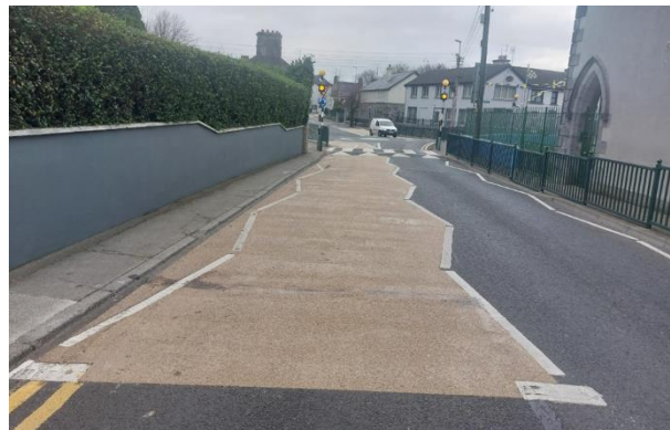
LOW-COST SAFETY IMPROVEMENT WORKS AT APPROACHES TO MINI ROUNDABOUT AT BARRACK ST. LOUGHREA
